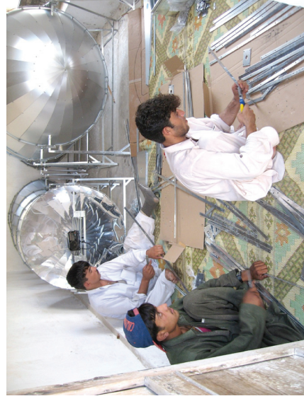
"workshop for future" - young men learning how to construct solar-oven and solar-lamps
